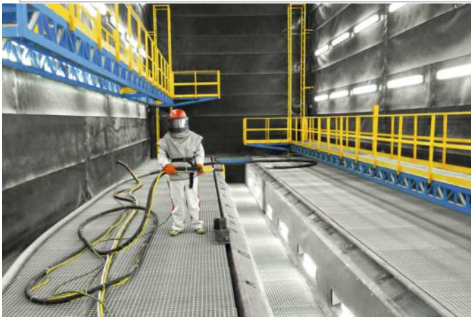
Blast rooms with lifting platforms
