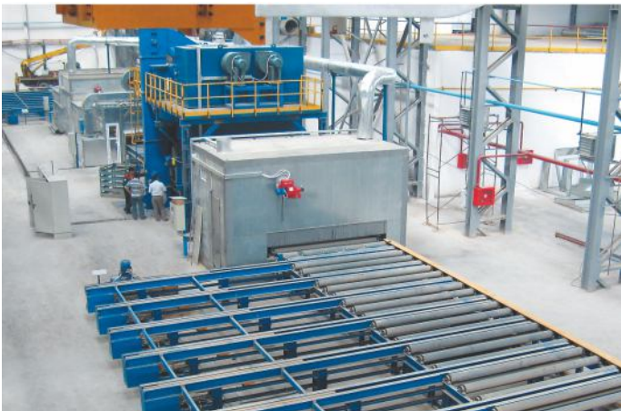
Shot blasting and preservation line
