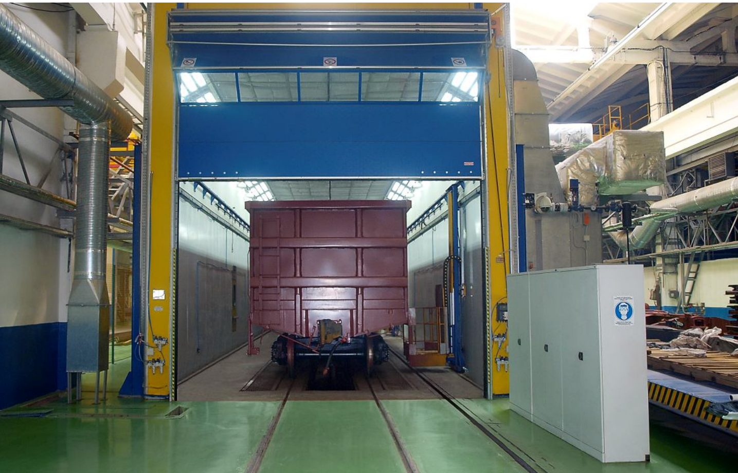
Painting and drying booth for wagons
