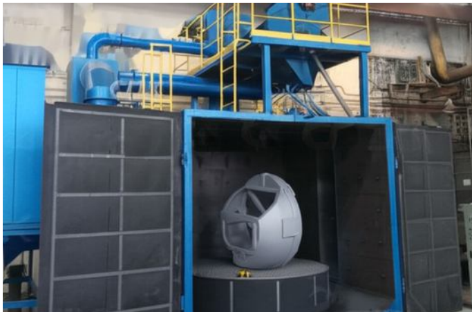
Shotblasting chamber with a turntable
